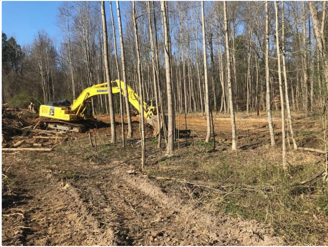
Figure 11: Clearing land for bridge foundations near I-40 and U.S. 401, December 2019 (photo: Spectrum News Staff)
